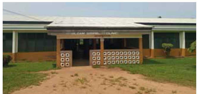
The clinic roof has now been completely replaced with new timber and metal sheets which have been painted white. Siloam supporters' generous gifts of £17,000 provided the funds for this major refurbishment by January 2023.
